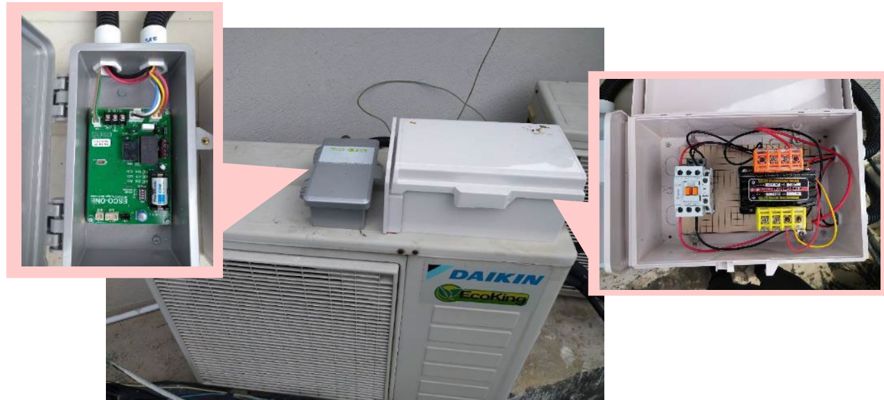
The outdoor unit with cyclic control
