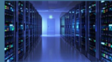
Cloud data center
